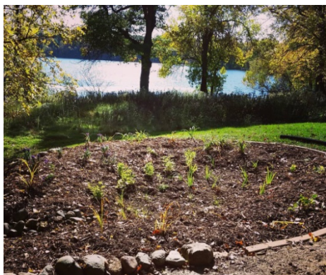
Left: A newly installed raingarden at Lakeridge of Woodbury Townhomes near Carver Lake, October 2016.
