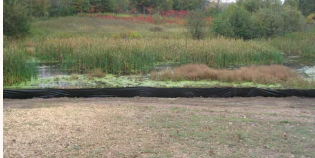
Properly-installed erosion control measures, such as silt fencing shown above, protect the adjacent water bodies from becoming polluted with eroded soil and chemicals. (SOURCE: WCD)
